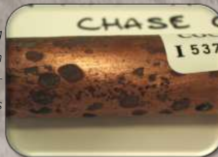
severe pitting corrosion on buried copper water lines
