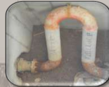
severe corrosion of buried firewater line
