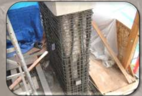
cathodic protection of a building support structure
